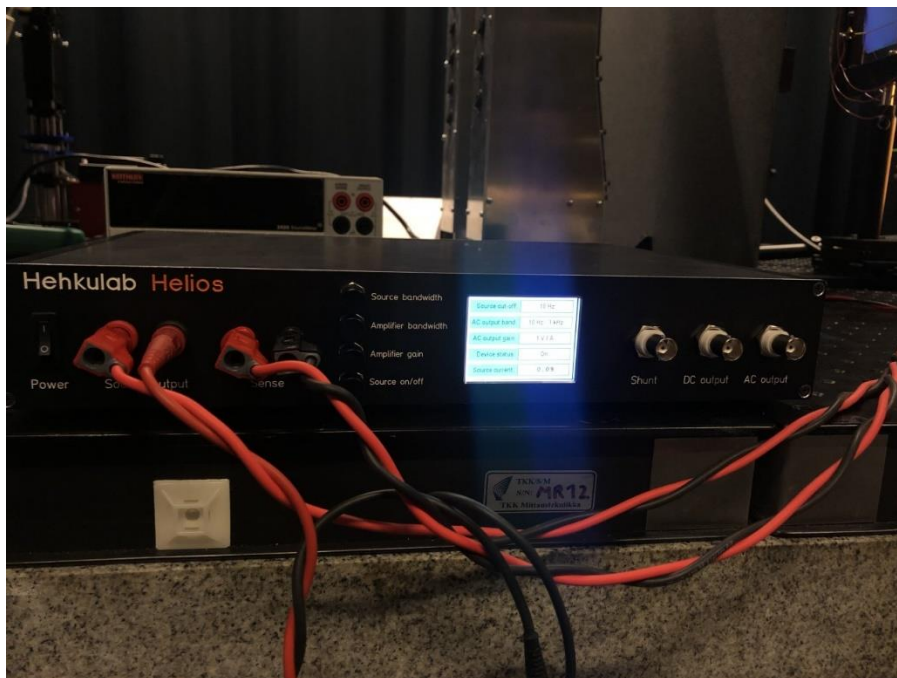
Figure 8: Hehkulab Helios connected to control the cell.
