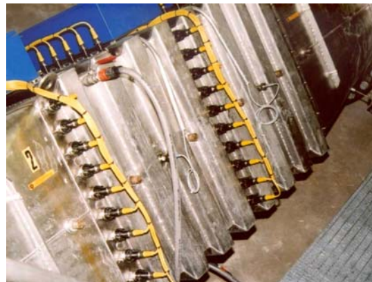
Figure 1a (top) UV-disinfection plants in water work Pitkälkoski/Helsinki, Finland. Figure 1b (bottom) several plant sensors can be seen at the side of the UV-plant.
